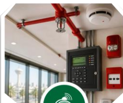
Fire Detection & Life Safety Systems
