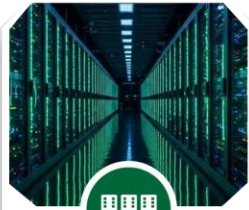
Data Center Infrastructure
