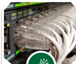
Fiber Optic & Structured Cabling Systems
